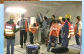
Construction work undertaken at Jinshazhou (金沙洲) Tunnel of Wuhan Guangzhou High Speed Rail.
